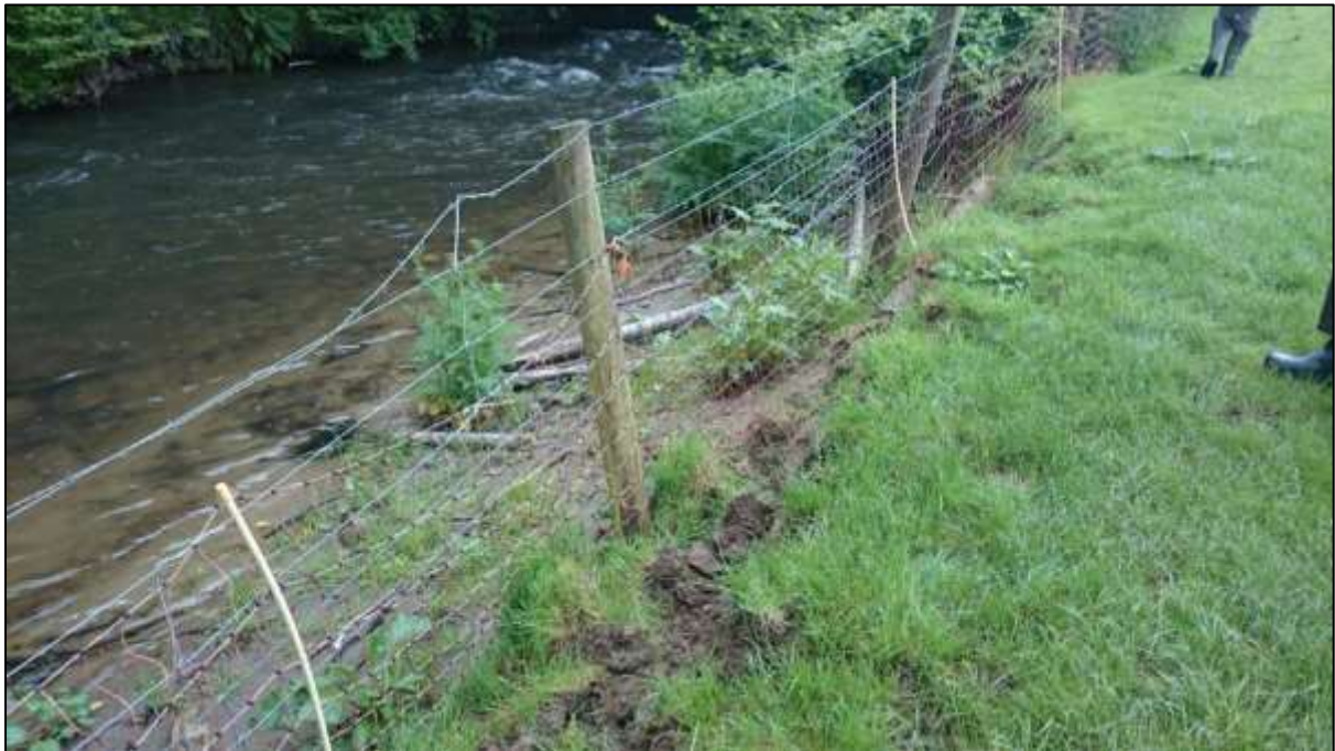
Figure 4: The fence line on the LB is situated very close to the river
