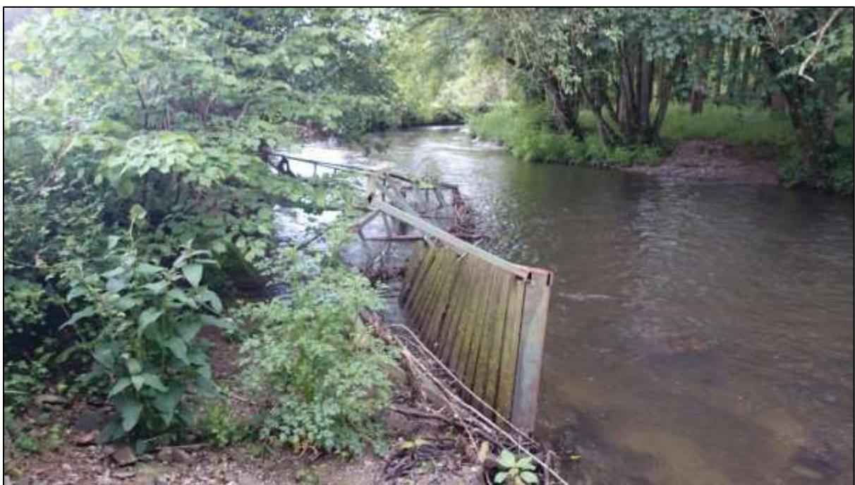
Figure 5: Powerful spate flows have destroyed a steel footbridge
